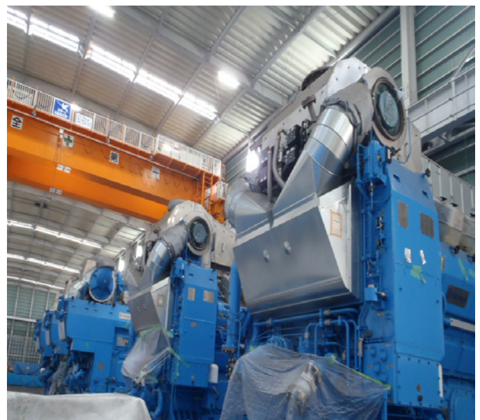
STARTERS OF COGENERATION ENGINES
